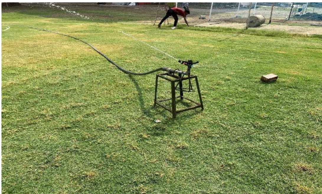
Figure: - Technology for Sprinkler system for gardening area.
